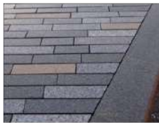
General paving to Footpaths: Caithness stone paving slabs 250mm/500mm wide x random lengths x 60mm thick.
