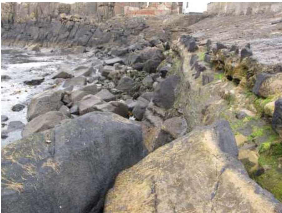
Image 1.3 – Loss of rock armour at root of the structure and exposed down stand beam
