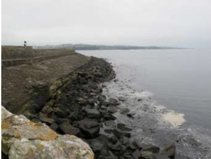
Image 1.1 – Typical view of breakwater and pitched revetment from the root of the structure
