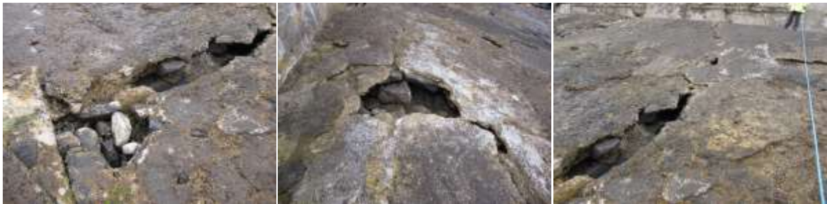
Image 1.2 – Deterioration of concrete overlay to stone pitched revetment, (multiple locations)
