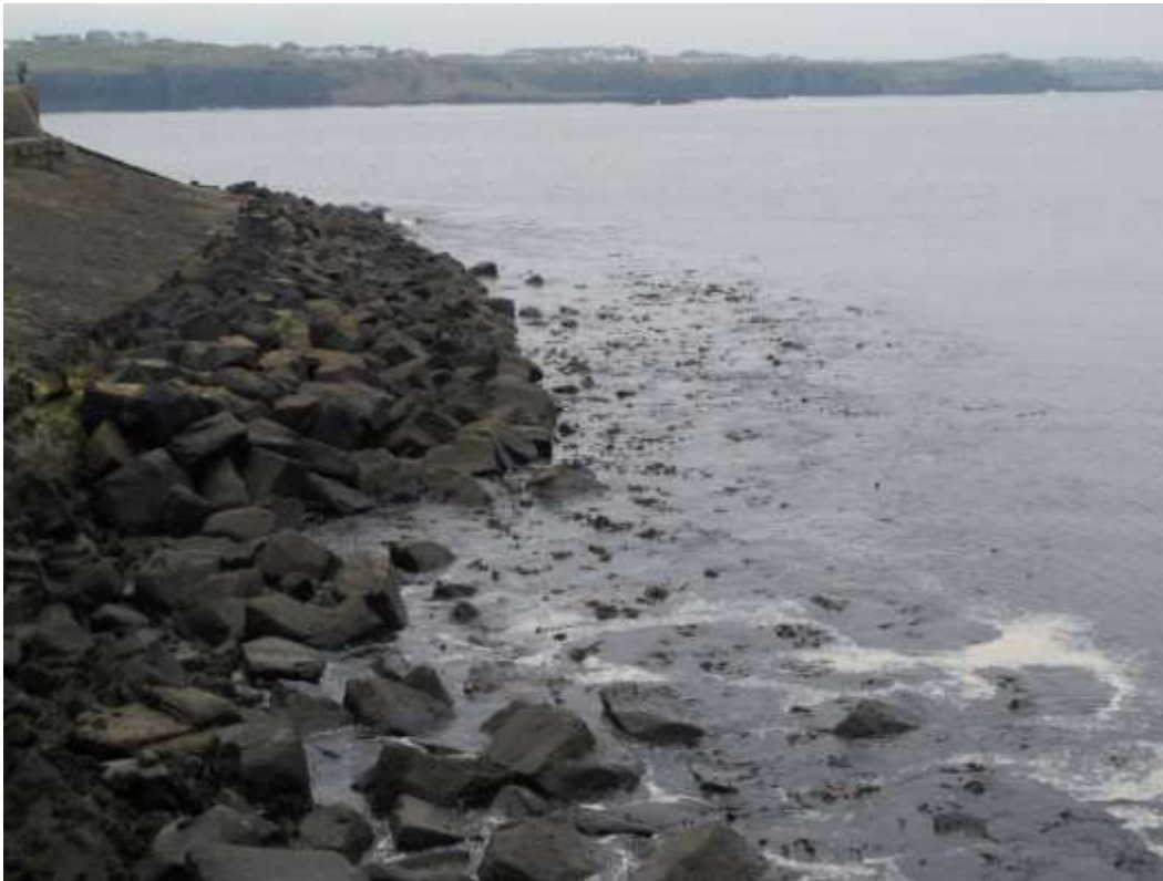
Image 1.4 – Loss of rock armour adjacent to sloping revetment
