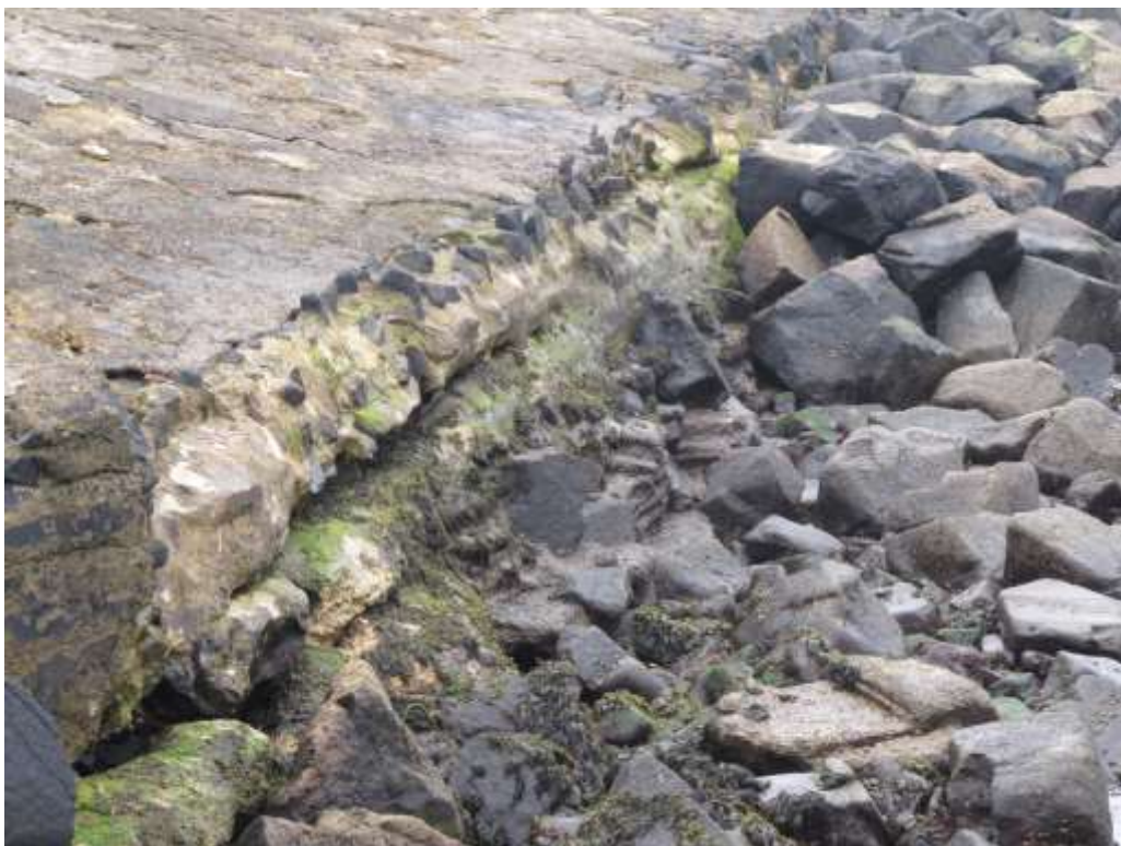
Image 1.5 – Deterioration of exposed down stand beam at root of structure
