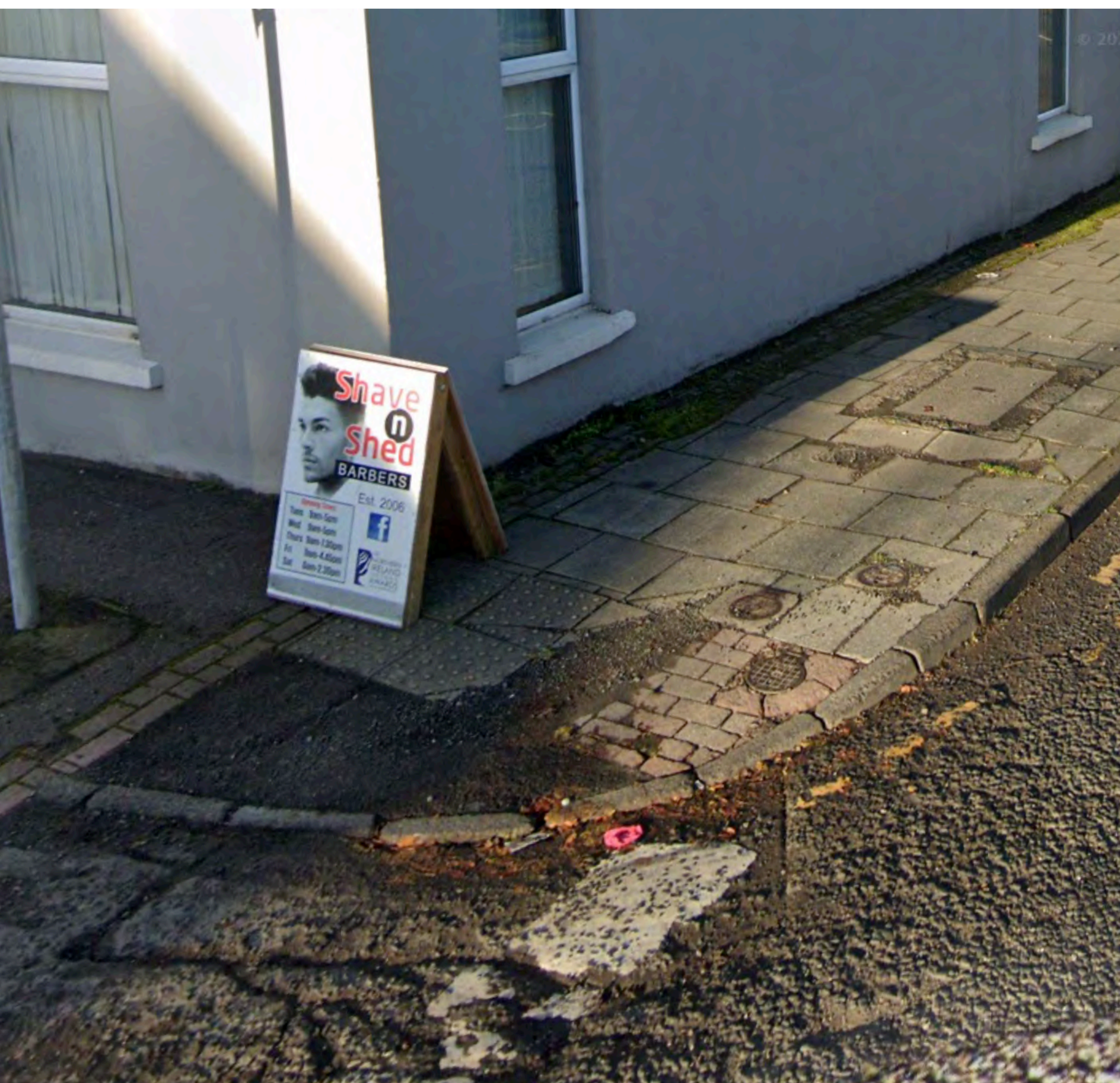
Current Condition - Uneven surfaces and trip hazards.
