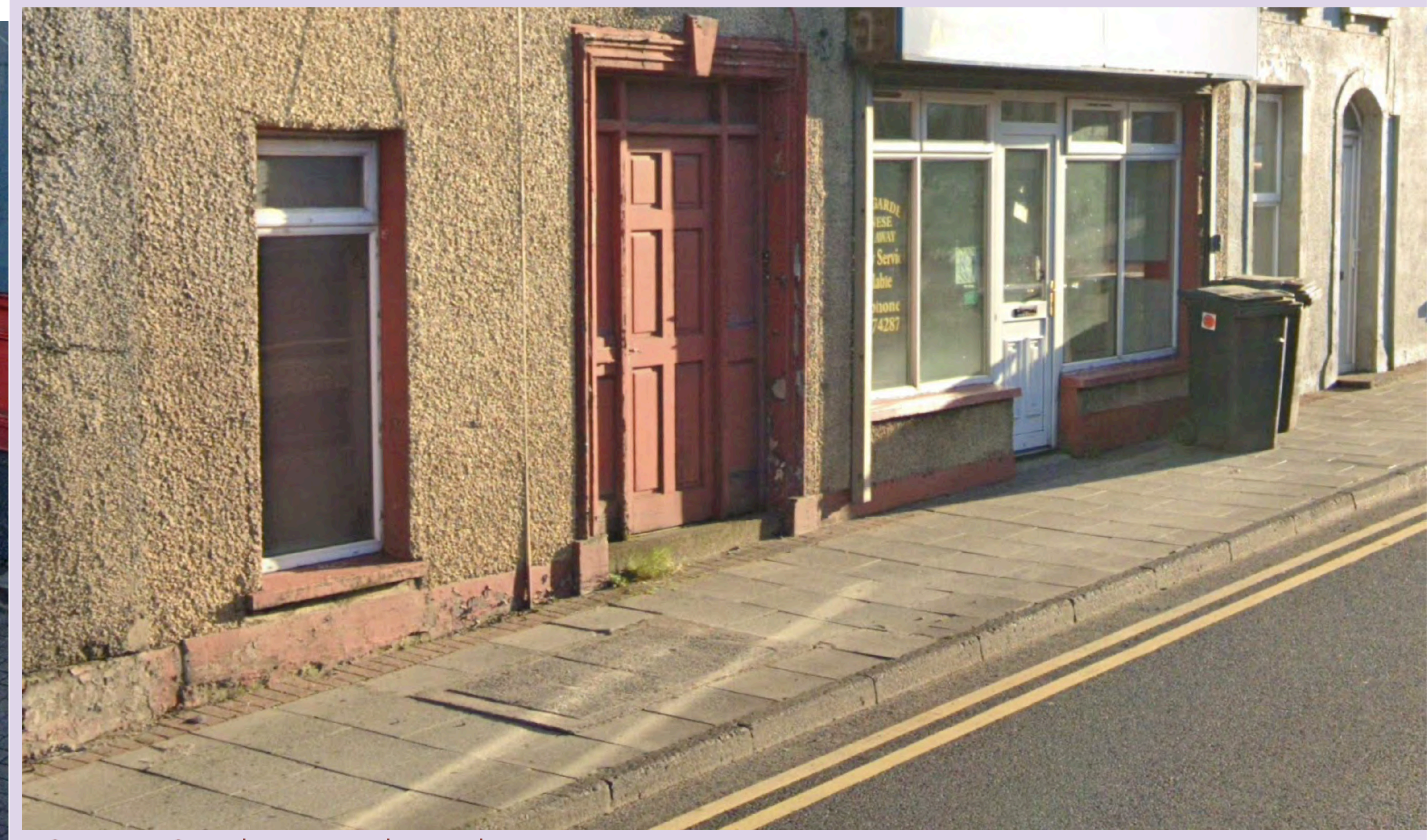
Current Condition trip hazard.
